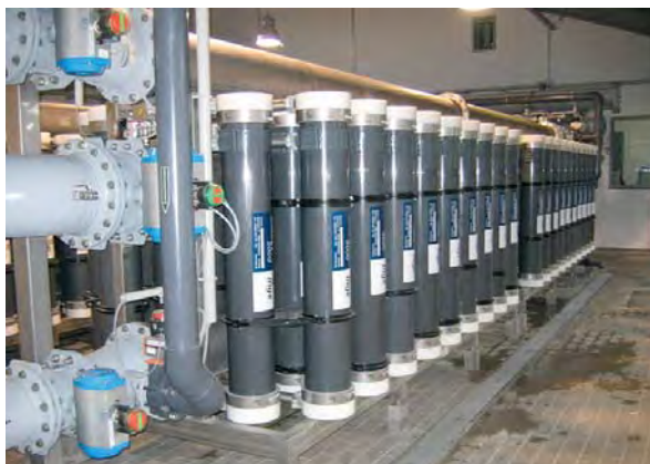
Ultrafiltration units for treating drinking water (stage 1)
